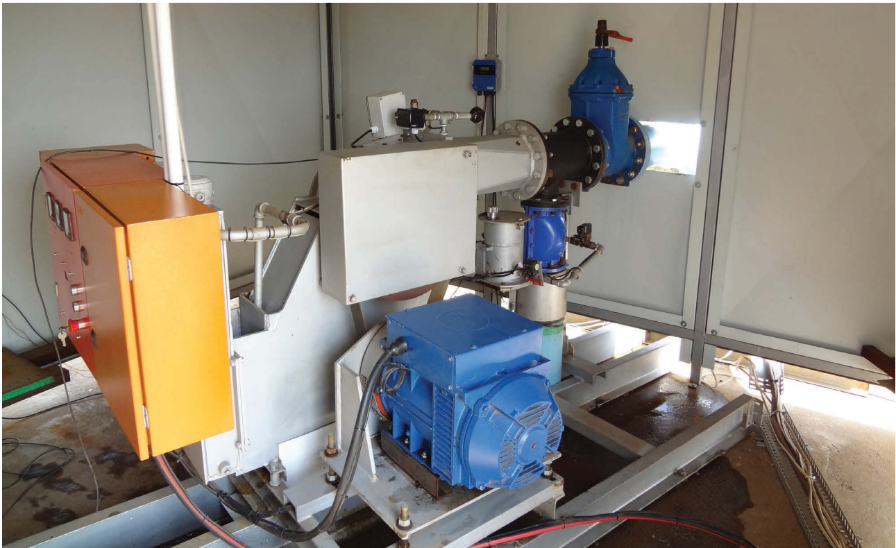
→ The conduit hydropower plant at the City of Tshwane, which generates power to be used for lighting, alarm systems and communication.
