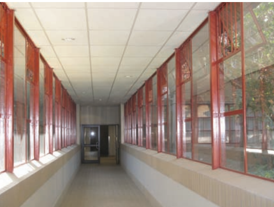
The passage between the two parts of the Aldoel Building which is accessible to persons with disabilities
