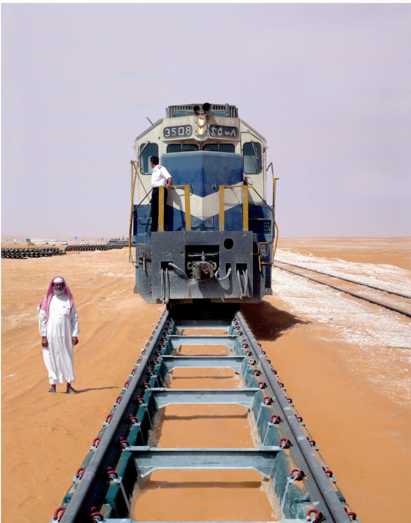
→ Tubular modular track constructed under extreme desert conditions in Saudi Arabia (photograph courtesy of tubular track).
