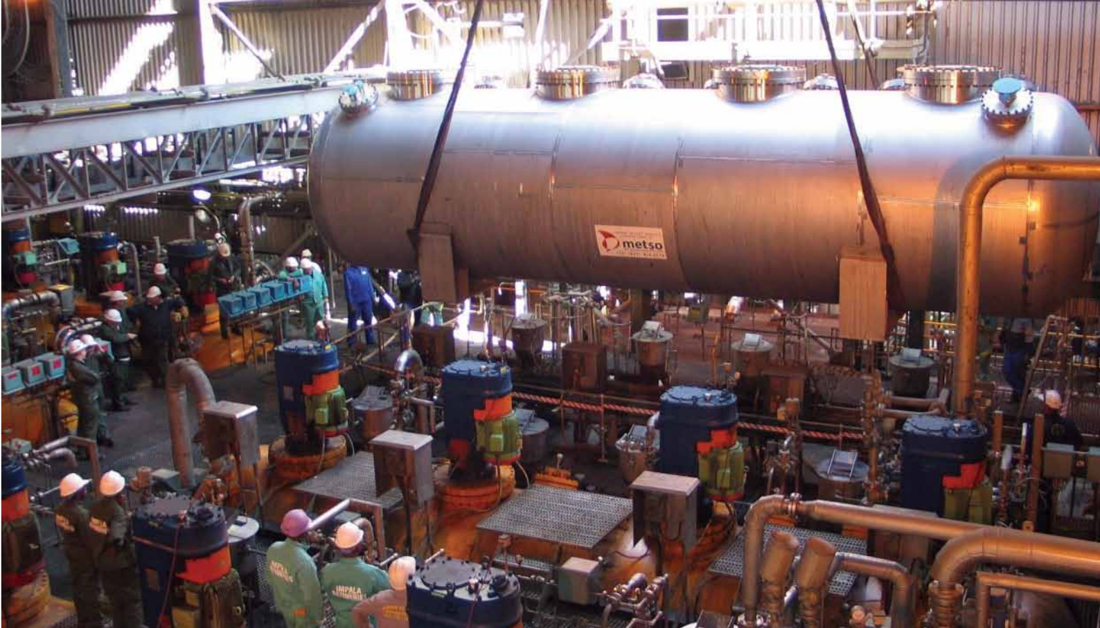
→ Installation of the completed second-stage leach autoclave at the BMR in June 2007.
