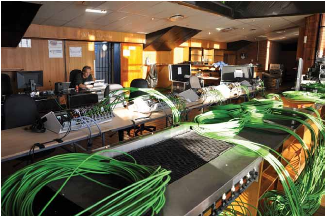
→ A commentary control room identical to the ones used during the FIFA 2010 Soccer World Cup.
