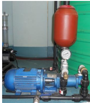
FIGURE 3.2: POSITIVE DISPLACEMENT PUMP AND ACCUMULATOR
