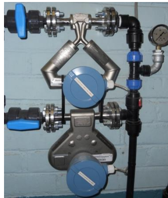
FIGURE 3.22: CORIOLIS FLOW METERS
